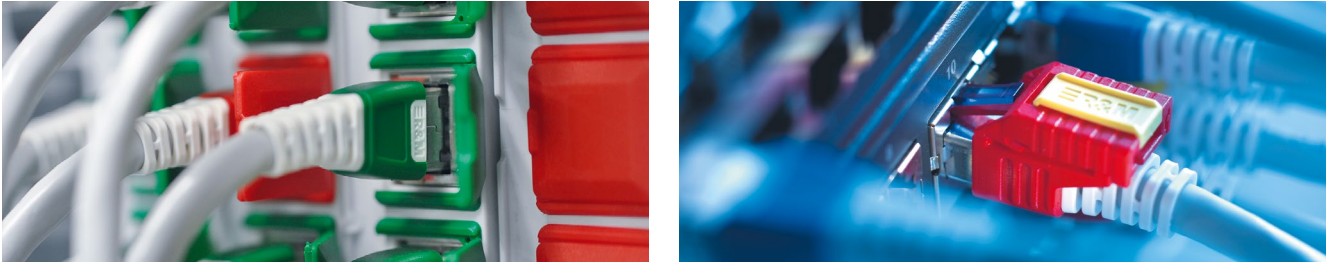
Security solutions from R&M, ranging from insertable color coded units (left) to locks for patch cords (right)
