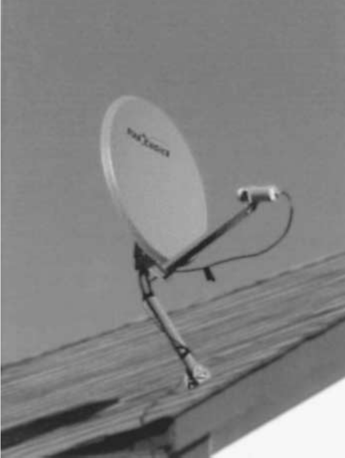
Figure 16.6 A typical DBS antenna installation.
