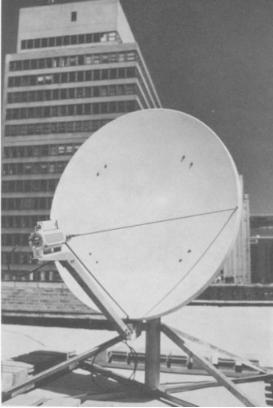
Figure 1.21 Photograph of the outdoor unit of a VSAT station. (Reproduced by permission of Gilat Satellite Networks, Ltd.)
