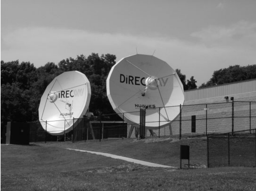
Figure 1.25 Photograph of the outdoor unit of a hub station. (Reproduced by permission of Hughes Network Systems, Inc.)
